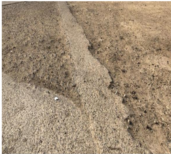
Figure 8. Rutting (Location No.3)
