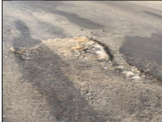
Figure 6. Pothole (Location No.3)
