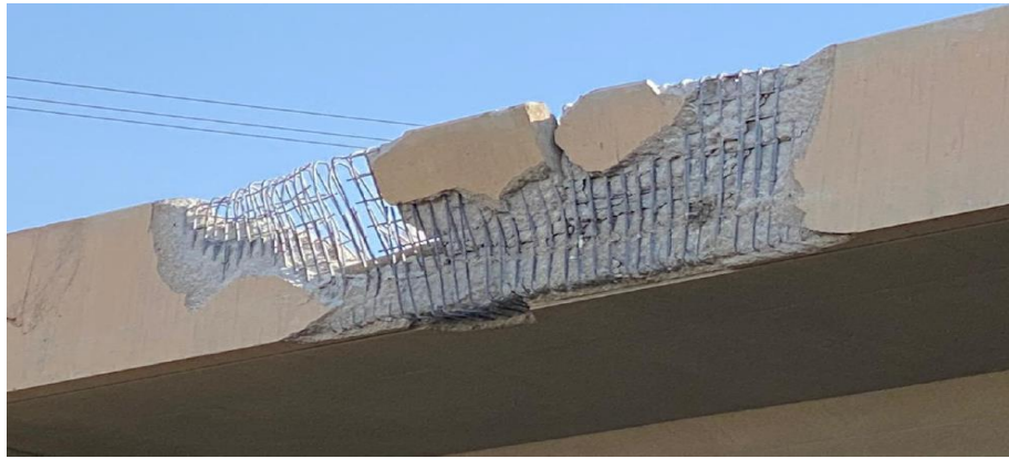
Figure 1: Damage caused to the Parapet of Bridge B02-0009 (B4929) Located at the Eastern Province, Rout 615, King Abdul-Aziz Road.
