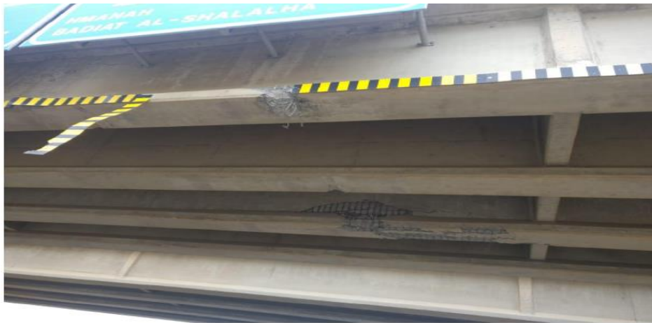
Figure 2: Damage caused to the Bridge Number B3429 Located at the Western Province, Rout 15, Makkah – Madinah Road.
